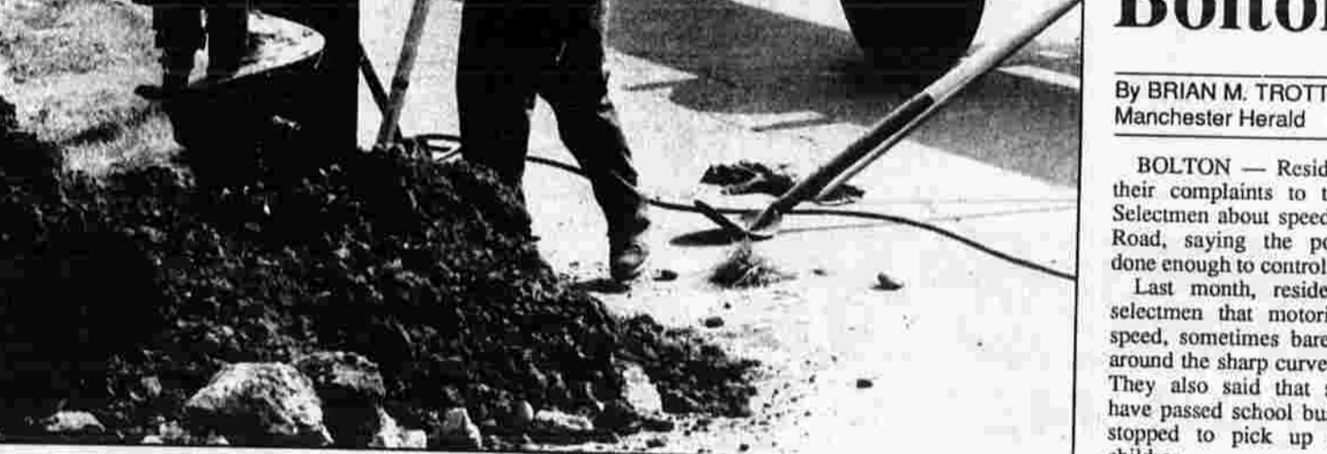
HARD WORK — Gil Olson, a worker for the contracting firm F.E. Hazard Ltd., works installing new utility poles throughout Manchester for Northeast Utilities.
